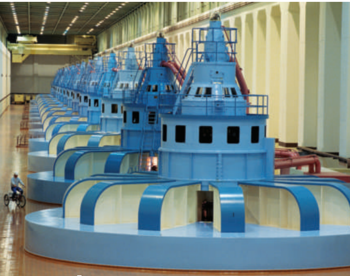
generators inside a hydroelectric power plant
